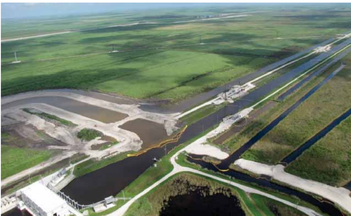
STA-1W Outflow Pump Station G-310 with structures and canals being constructed as part of STA-1W Expansion #1, looking northwest (photo by SFWMD, May 2018).
